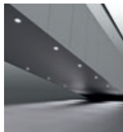
Soffit LED spot cladding lighting
